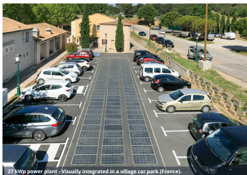
27 kWp power plant - Visually integrated in a village car park (France).
