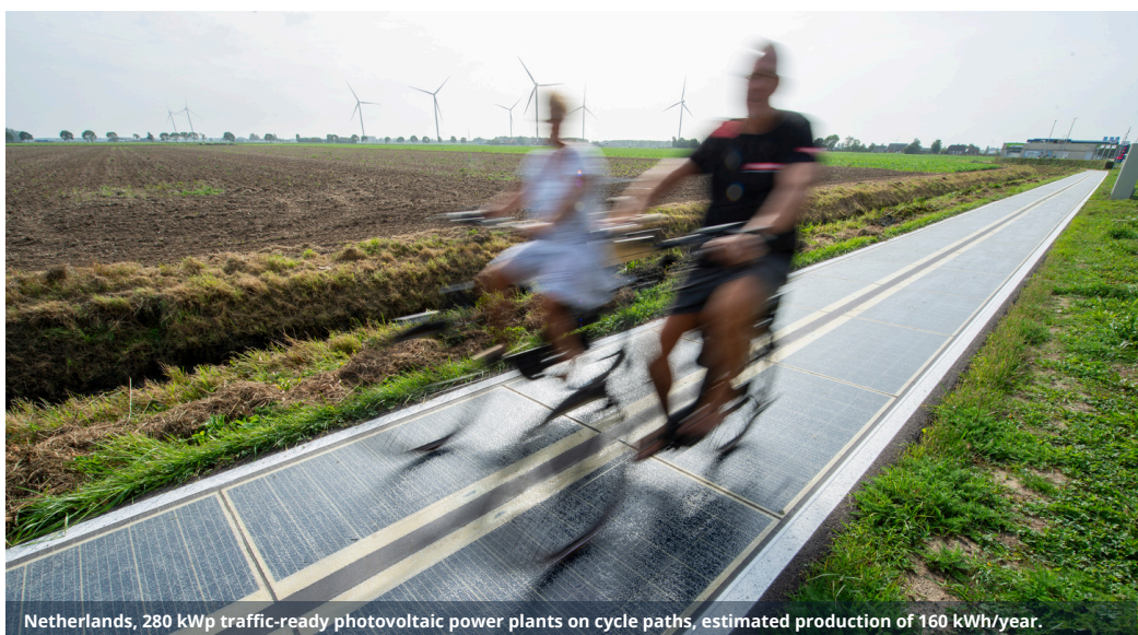
Netherlands, 280 kWp traffic-ready photovoltaic power plants on cycle paths, estimated production of 160 kWh/year.
